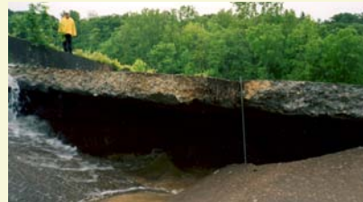
Dam Spillway Failure
